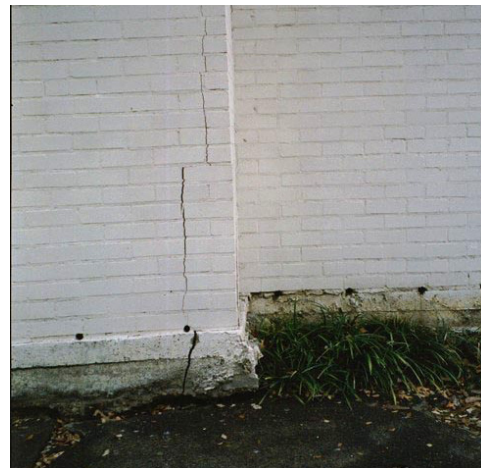
Fig. 8 Cracked foundation on home due to the shrinking and swelling of Houston Black clay it was built upon. Credit: Clay Robinson
